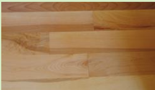
Too-Close End Joints
